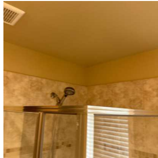
Exhaust Vent (11/16) 08/02/2024 2:05 PM
