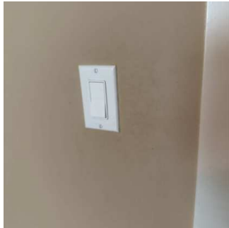
Power Outlets (10/16) 08/02/2024 1:55 PM
