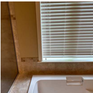
Exhaust Vent (13/16) 08/02/2024 2:05 PM
