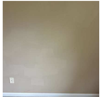
Power Outlets (16/16) 08/02/2024 1:40 PM
