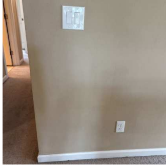
Power Outlets (10/16) 08/02/2024 1:40 PM
