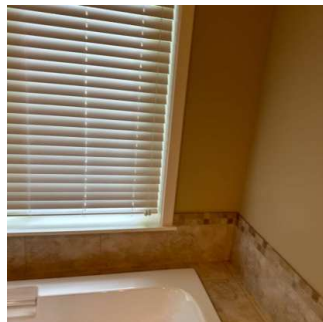
Exhaust Vent (15/16) 08/02/2024 2:05 PM
