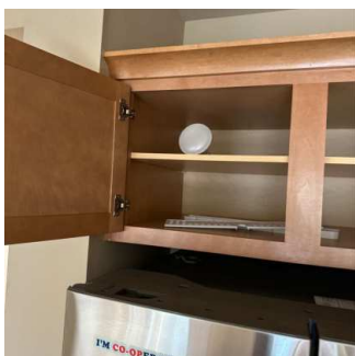
Power Outlets (13/16) 08/02/2024 1:22 PM
