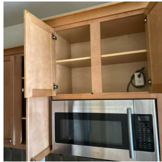
Power Outlets (7/16) 08/02/2024 1:22 PM
