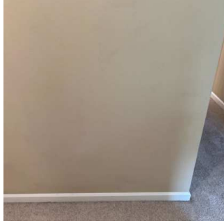
Power Outlets (7/16) 08/02/2024 1:40 PM
