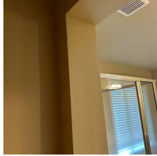
Exhaust Vent (7/16) 08/02/2024 2:05 PM
