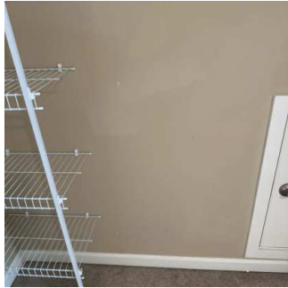
Power Outlets (7/16) 08/02/2024 1:55 PM
