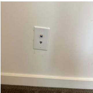
Switches / outlets / wall plates continued (3/16) 08/01/2024 1:30 PM
