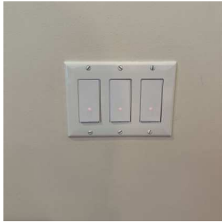
Switches / outlets / wall plates continued 2 (8/16) 08/01/2024 1:35 PM
