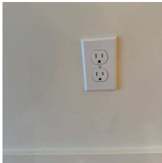
Switches / outlets / wall plates continued (16/16) 08/01/2024 1:34 PM
