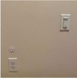
Switches / outlets / wall plates continued 2 (11/16) 08/01/2024 1:35 PM
