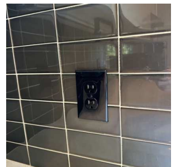
Switches / outlets / wall plates continued 2 (6/16) 08/01/2024 1:35 PM
