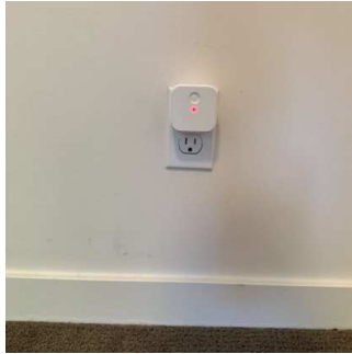
Switches / outlets / wall plates continued 2 (13/16) 08/01/2024 1:36 PM
