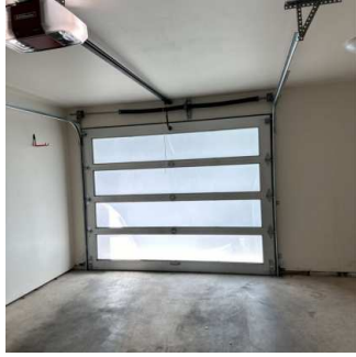
Garage Doors / Openers (2/2) 08/01/2024 2:28 PM
