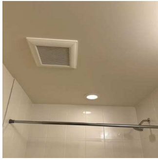
Light fixtures (6/16) 08/01/2024 1:51 PM
