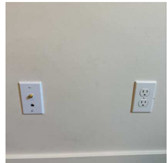
Outlets continued (2/8) 08/01/2024 1:36 PM
