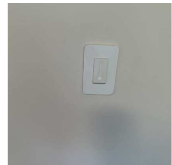
Switches / Outlets / Wall Plates (4/16) 08/01/2024 1:29 PM
