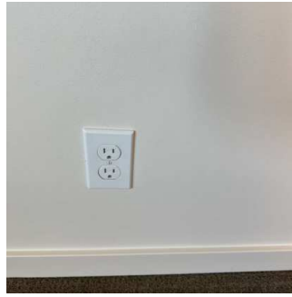
Switches / Outlets / Wall Plates (7/16) 08/01/2024 1:29 PM
