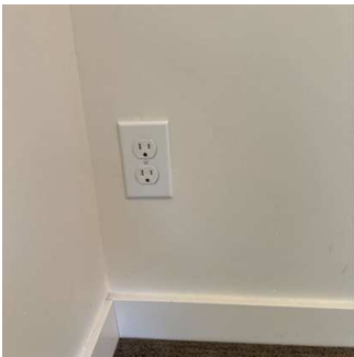
Switches / outlets / wall plates continued 2 (15/16) 08/01/2024 1:36 PM
