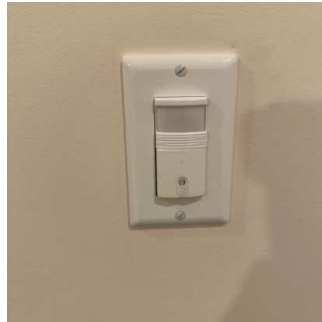
Switches / Outlets / Wall Plates (15/16) 08/01/2024 1:30 PM
