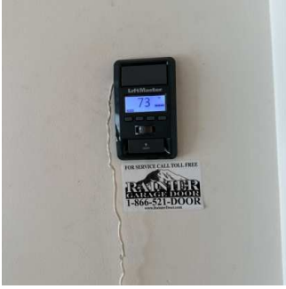
Garage Doors / Openers (1/2) 08/01/2024 2:28 PM
