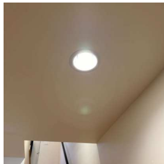
Light fixtures (3/16) 08/01/2024 1:51 PM
