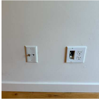
Switches / outlets / wall plates continued (12/16) 08/01/2024 1:34 PM
