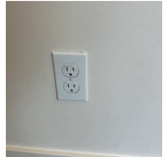
Switches / outlets / wall plates continued (2/16) 08/01/2024 1:30 PM
