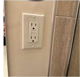
Switches / Outlets / Wall Plates (12/16) 08/01/2024 1:29 PM
