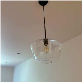
Light fixtures (13/16) 08/01/2024 1:53 PM
