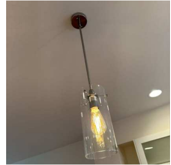
Light fixtures (12/16) 08/01/2024 1:53 PM
