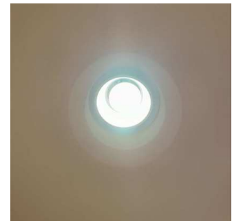
Light fixtures (4/16) 08/01/2024 1:51 PM
