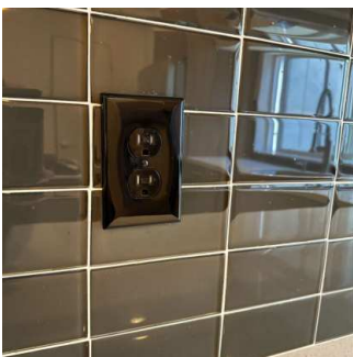
Switches / outlets / wall plates continued 2 (3/16) 08/01/2024 1:35 PM
