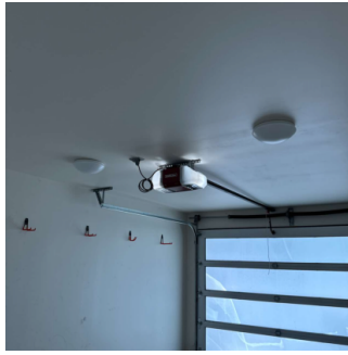
Light fixtures (7/16) 08/01/2024 1:52 PM
