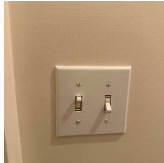
Switches / Outlets / Wall Plates (14/16) 08/01/2024 1:29 PM
