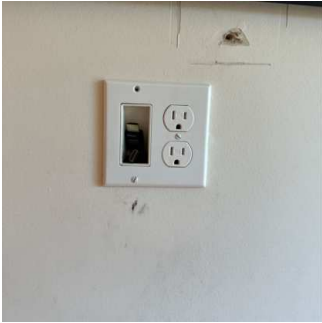
Switches / outlets / wall plates continued (11/16) 08/01/2024 1:34 PM
