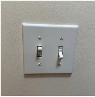
Switches / outlets / wall plates continued (7/16) 08/01/2024 1:30 PM
