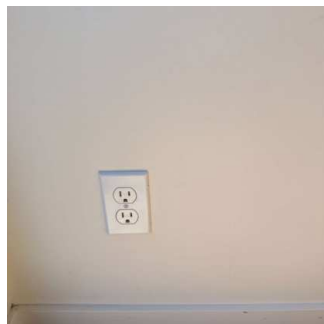
Switches / Outlets / Wall Plates (2/16) 08/01/2024 1:28 PM
