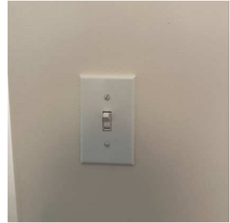
Switches / outlets / wall plates continued 2 (14/16) 08/01/2024 1:36 PM
