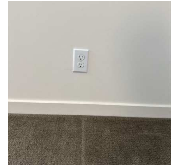
Switches / Outlets / Wall Plates (8/16) 08/01/2024 1:29 PM
