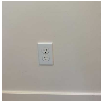
Switches / outlets / wall plates continued 2 (16/16) 08/01/2024 1:36 PM
