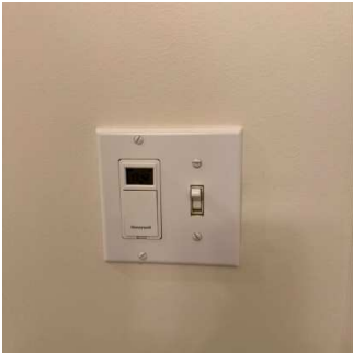
Switches / Outlets / Wall Plates (13/16) 08/01/2024 1:29 PM
