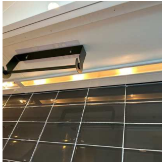
Light fixtures (15/16) 08/01/2024 1:53 PM
