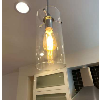
Light fixtures (11/16) 08/01/2024 1:53 PM
