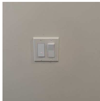
Switches / Outlets / Wall Plates (3/16) 08/01/2024 1:29 PM
