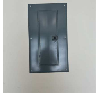
Electrical Panel (1/3) 08/01/2024 1:59 PM
