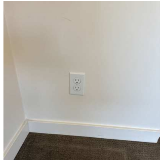
Switches / Outlets / Wall Plates (6/16) 08/01/2024 1:29 PM
