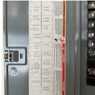
Electrical Panel (3/3) 08/01/2024 1:59 PM
