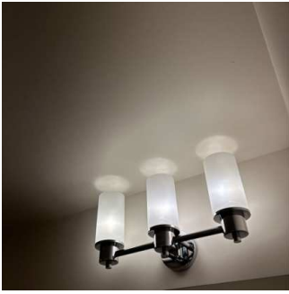
Light fixtures (5/16) 08/01/2024 1:51 PM
