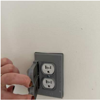
Outlets continued (7/8) 08/01/2024 1:37 PM
