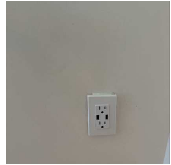
Switches / outlets / wall plates continued (14/16) 08/01/2024 1:34 PM
