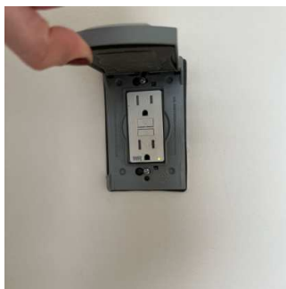
Outlets continued (5/8) 08/01/2024 1:37 PM
