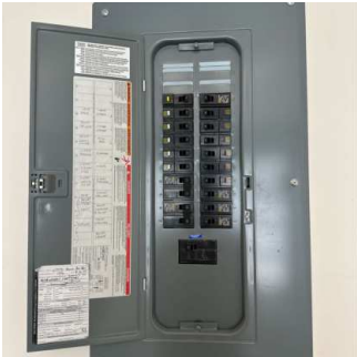
Electrical Panel (2/3) 08/01/2024 1:59 PM
