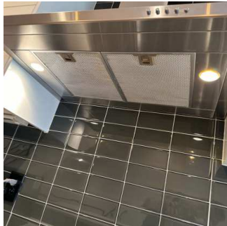
Light fixtures (14/16) 08/01/2024 1:53 PM
