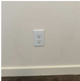
Outlets continued (1/8) 08/01/2024 1:36 PM
