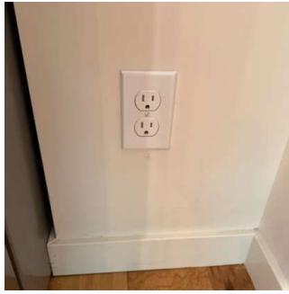
Switches / outlets / wall plates continued 2 (9/16) 08/01/2024 1:35 PM
