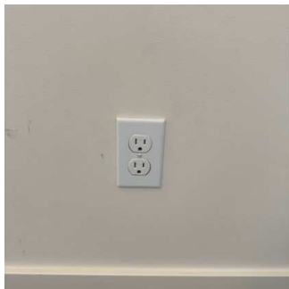
Switches / outlets / wall plates continued (4/16) 08/01/2024 1:30 PM
