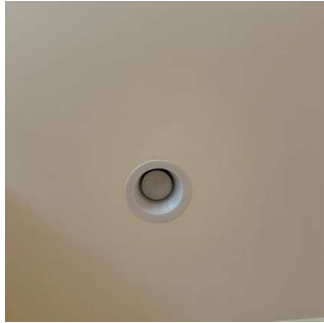
Light fixtures (10/16) 08/01/2024 1:52 PM
