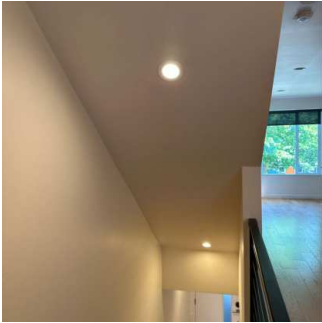
Light fixtures (9/16) 08/01/2024 1:52 PM
