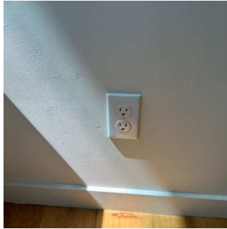
Switches / outlets / wall plates continued (13/16) 08/01/2024 1:34 PM
