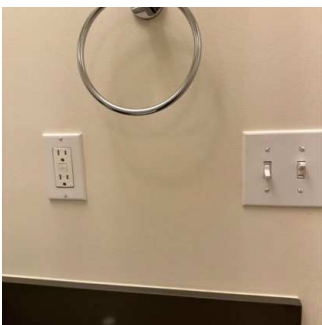
Outlets continued (3/8) 08/01/2024 1:36 PM
