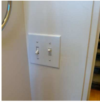
Switches / outlets / wall plates continued (9/16) 08/01/2024 1:31 PM
