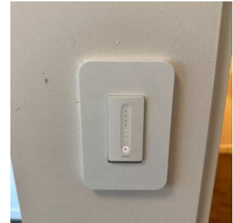
Switches / Outlets / Wall Plates (16/16) 08/01/2024 1:30 PM
