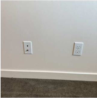
Switches / Outlets / Wall Plates (9/16) 08/01/2024 1:29 PM
