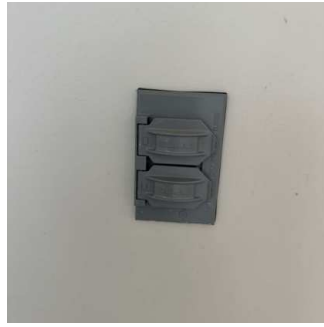
Outlets continued (8/8) 08/01/2024 1:37 PM
