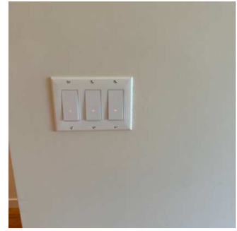
Switches / outlets / wall plates continued (10/16) 08/01/2024 1:34 PM
