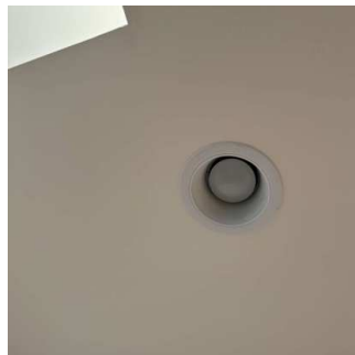
Light fixtures continued (13/16) 08/01/2024 1:55 PM
