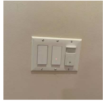
Switches / outlets / wall plates continued 2 (10/16) 08/01/2024 1:35 PM
