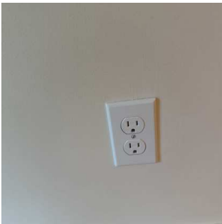
Switches / outlets / wall plates continued (15/16) 08/01/2024 1:34 PM
