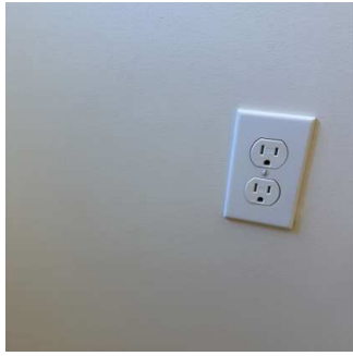
Switches / outlets / wall plates continued (8/16) 08/01/2024 1:31 PM
