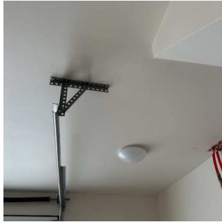
Light fixtures continued 2 (5/5) 08/01/2024 1:59 PM
