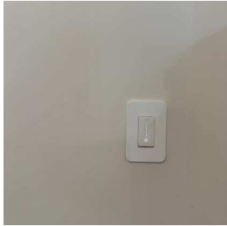
Switches / outlets / wall plates continued 2 (12/16) 08/01/2024 1:35 PM
