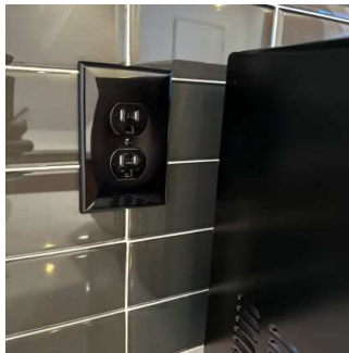
Switches / outlets / wall plates continued 2 (1/16) 08/01/2024 1:34 PM
