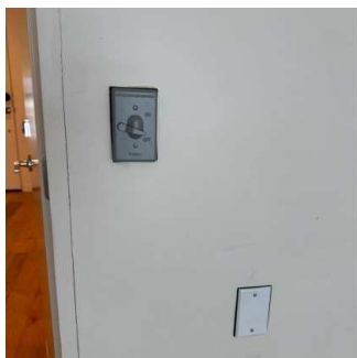
Outlets continued (4/8) 08/01/2024 1:36 PM
