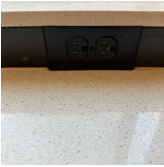
Switches / outlets / wall plates continued 2 (7/16) 08/01/2024 1:35 PM
